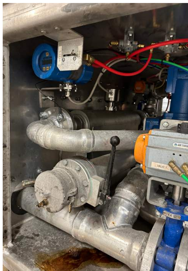
Truck-mounted TCM-65K Coriolis meter
