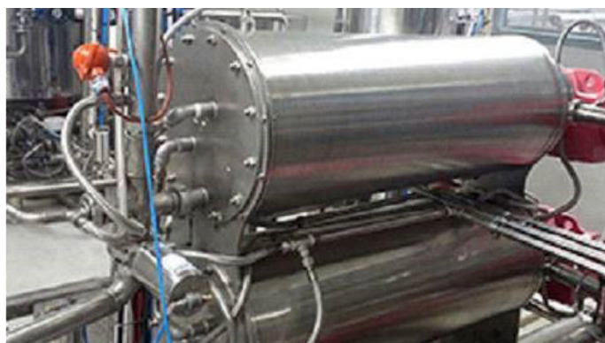
Mixing and aeration tanks where the product is mixed with air
