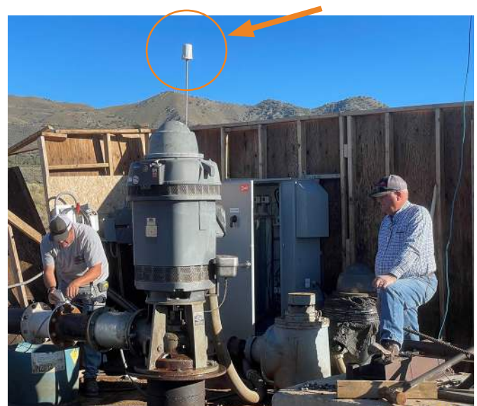
On this multi-generational farm, Marc's dad is making sure he gets the repair right. He, too, appreciates the benefits of the RANGER and the SignalFire Cloud. This is pump house #2 that a second RANGER is monitoring.
